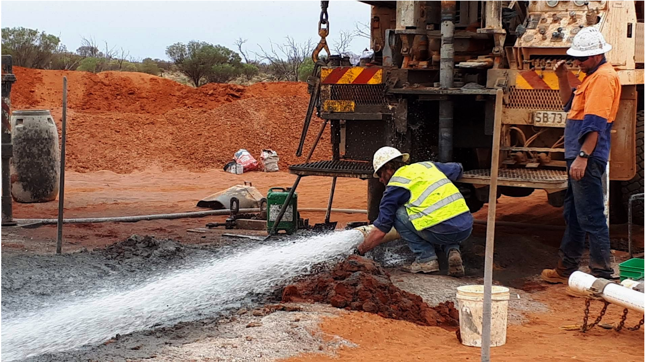
Figure 1: Underground water gushes out from new Bore Hole 1 at Aurora Tank
