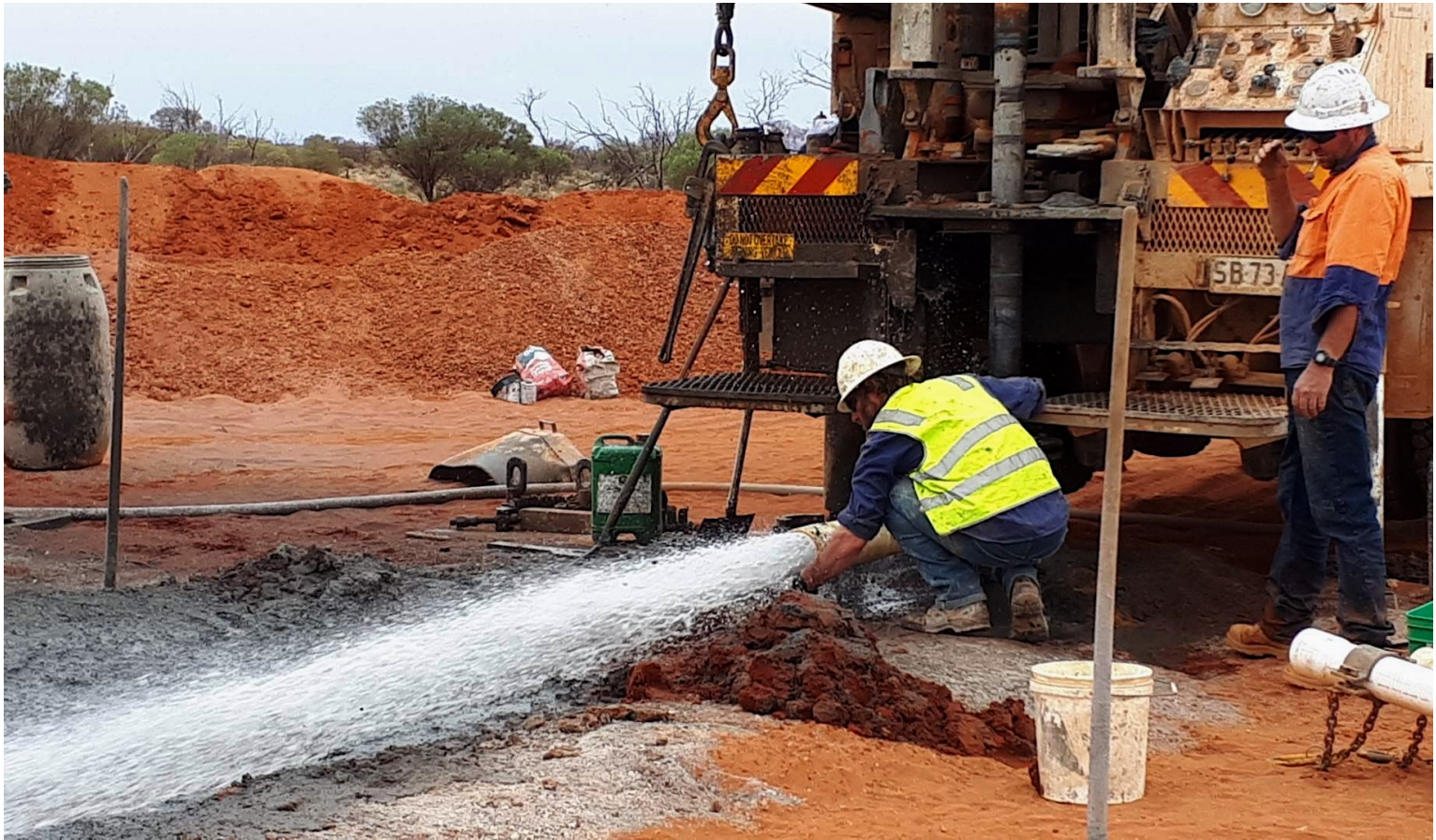
Figure 10: Marmota finds underground water source at Aurora Tank (Dec 2020)
